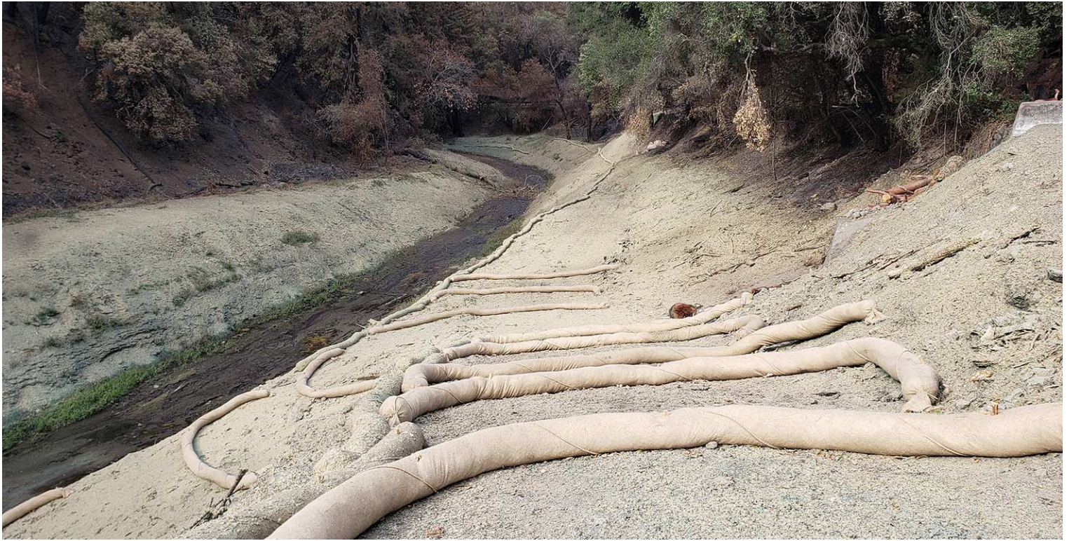
The newly constructed plane bed channel just after the Glass Fire swept through the site.
