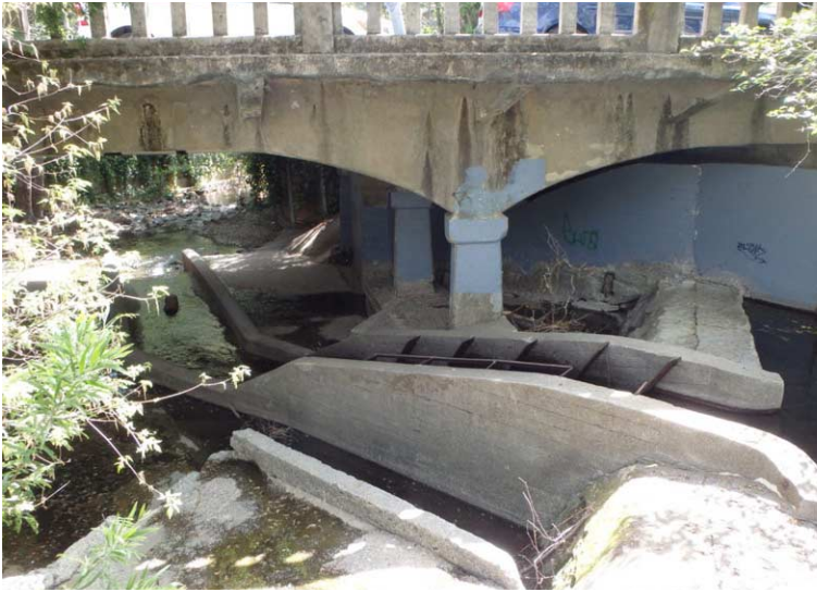
Removing fish passage barriers, such as this poorly functioning fish ladder, is a high priority for state and federal agencies. Photo courtesy Nicholas Brinton
