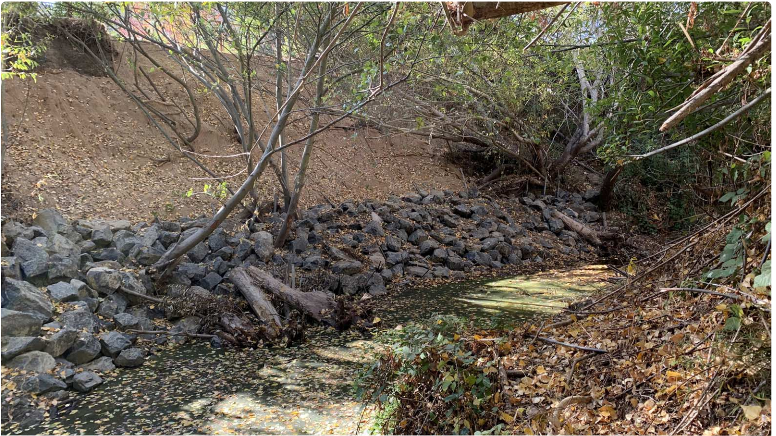
A hybrid approach using hard and soft engineering bank stabilization where riprap and pieces of wood were installed to stabilize the toe of the streambank. The upper portion was then laid back to a gentle slope, planted with willows, seeded with shade-tolerant native riparian species, and protected with a biodegradable coir erosion control blanket. Designed by Matt Smeltzer at geomorphDESIGN and constructed by Spye Construction. Photo courtesy Marin County DPW.
